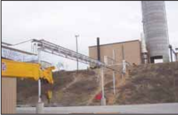
A.W. Stiles Contractors installed this new main steam line to kilns from a new boiler.
