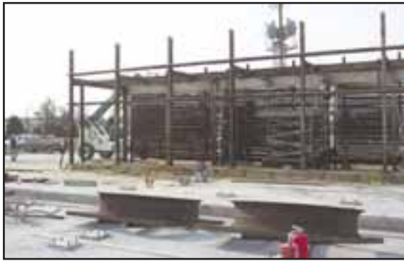
Employees of A.W. Stiles remove a track kiln in order to relocate it to another location.
