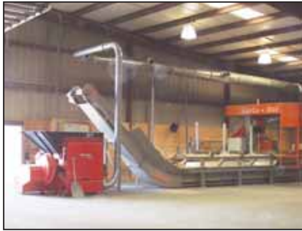
Atlanta Metro Lumber & Reload precision end trim saws lumber to specified lengths with a Holtec Precision Trim Saw upon request.
