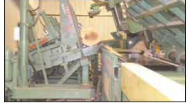
Yoder's carriage is manufactured by Cleereman with a 17-degree slant with 4-head blocks that is also used in combination with a USNR optimizer scanner.
