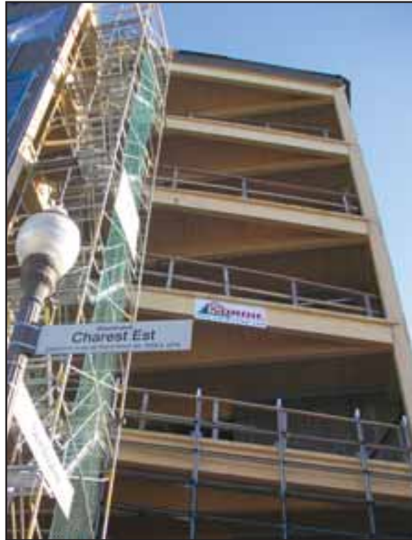
Made of Black Spruce glue laminated beams, columns and decking, the unique construction technology featured in this project is paving the way for similar alternative building projects across North America.
