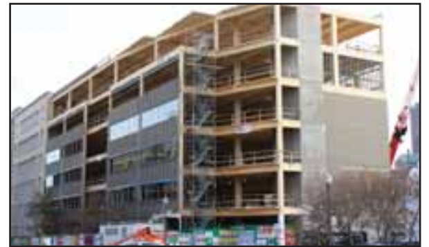
The six-story Fondation commercial structure, which features heavy timber frame construction designed and provided by Nordic Structures, is the first of its kind built in Canada.
