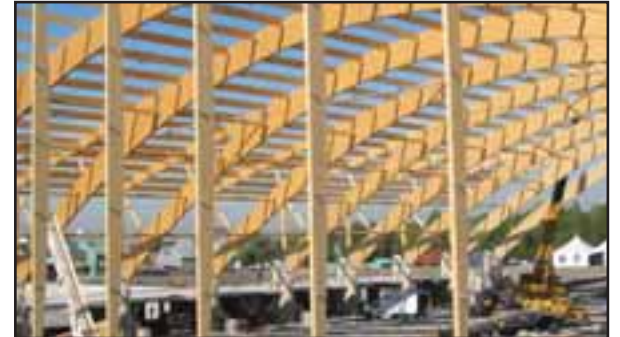
Nordic's Enviro=Lam used here in the construction of a sports complex. This soccer stadium features 210-foot clearspan glulam arches.
