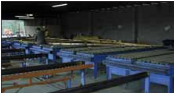
Members of the roof crew at work on the building and assembly of roof trusses
