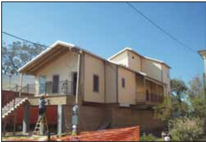
Pictured is a two-story Make-It-Right Foundation home in the Lower 9th Ward of New Orleans. Indiana Building Systems purchases approximately 2,500,000 board feet of lumber, specifically SYP and SPF, for the manufacture of various types of structures.
