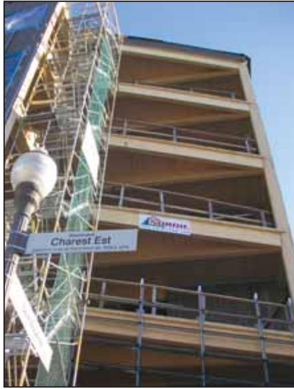
Made of Black Spruce glue laminated beams, columns and decking, the unique construction technology featured in this project is paving the way for similar alternative building projects across North America.
