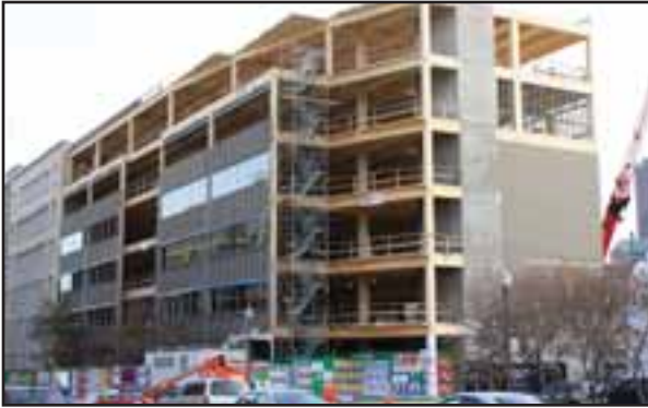
The six-story Fondation commercial structure, which features heavy timber frame construction designed and provided by Nordic Structures, is the first of its kind built in Canada.
