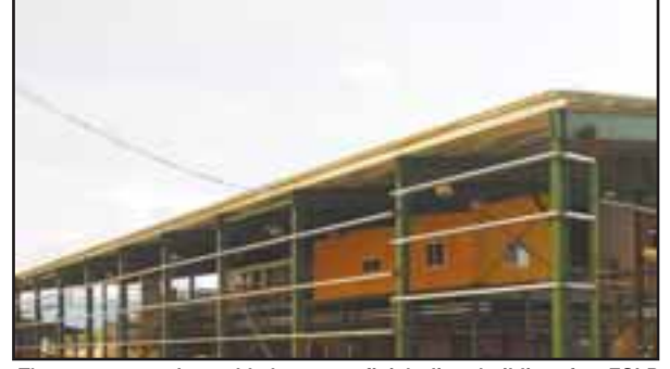
The company also added a new finish line building for ESLP (Engelmann Spruce-Lodgepole Pine) boards.
