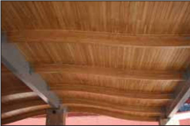
FILLER KING®/Boise Cascade curved glulam beams and laminated wood roof decking help beautify the Talking Sticks Casino in Phoenix, Ariz.
