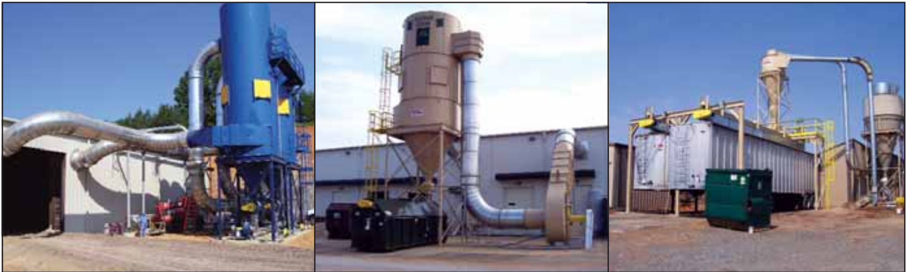
Southern Pneumatics Dust Collection Systems shown at different locations throughout the United States.
