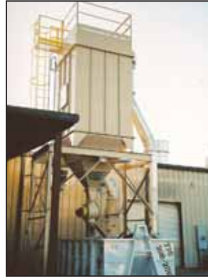
This Southern Pneumatics baghouse was installed at a custom cabinet shop in White, Ga.
