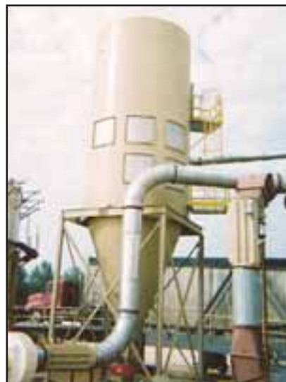
The company also installed this MAC baghouse at a composite flooring plant in Selma, Ala.
